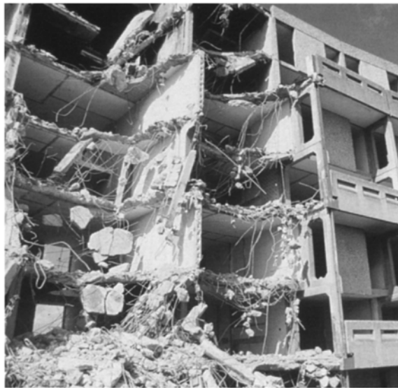
10.3 Barrie Crescent Hulme undergoing demolition. This example is typical of the balcony access, system built blocks.
