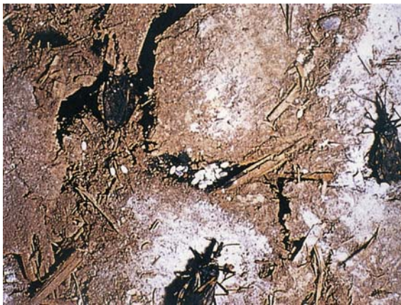
Plate 82: Cracks in the walls of the mud huts in poor rural areas are the favourite habitats of reduviid bugs.
