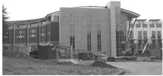
Figure 9.3 The new Lowes Corporate Headquarters under construction, 2003, Calloway Johnson Moore and West, architects. This refreshingly contemporary design is free from the needless neoclassical ornamentation so beloved by other North Carolina architects.
