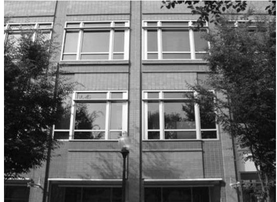
Figure 6.31 Gateway Village, Charlotte, NC, Duda Paine, architects, 2001, detail. The façade of this large office building is enriched by the subtle details of the brick and tile cladding, where small projections and recessions combine with changes of material to break down the surface into a complex grid of regulating lines.
