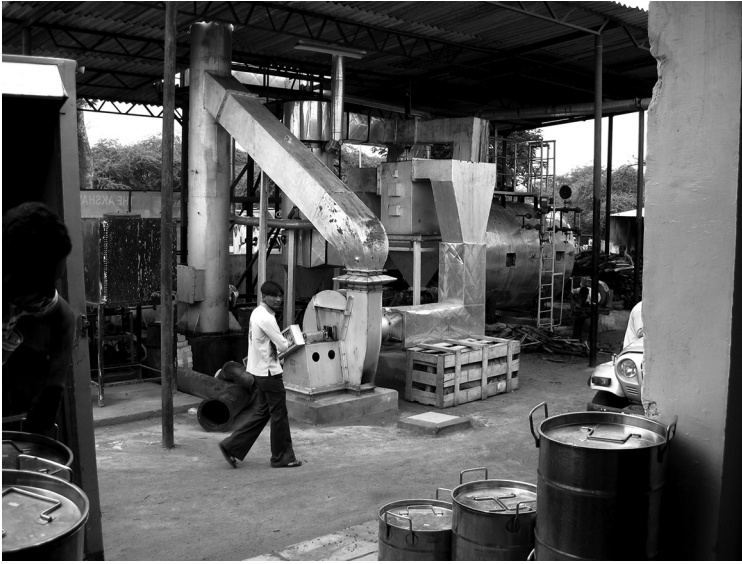
Figure A8.9 Boiler.
