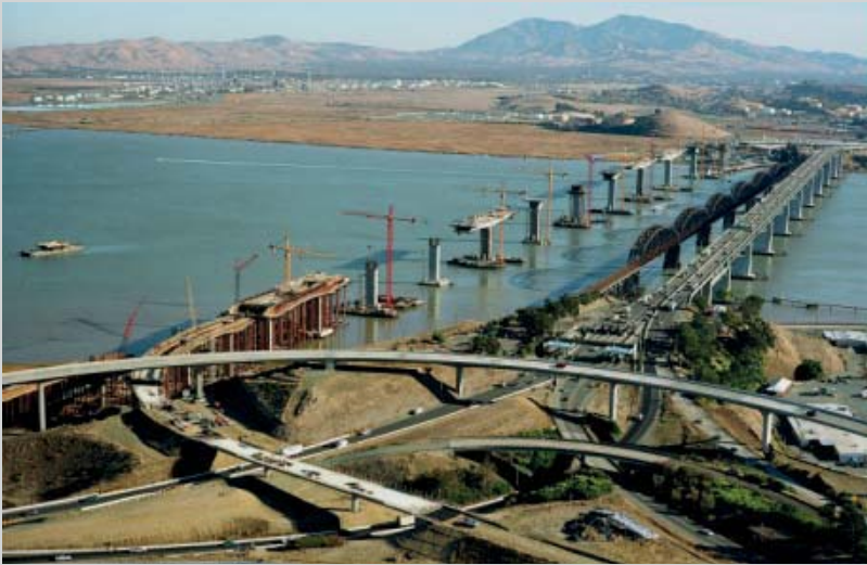
FIGURE 8.CS1 Benicia–Martinez Bridge under construction looking from Benicia, California (courtesy of Kiewit Infrastructure West).
