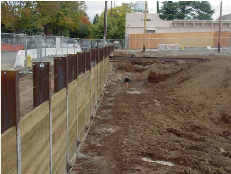
FIGURE 6.29 Soldier beam and lagging wall with tieback and no waler, Enloe Hospital, Chico, California.
