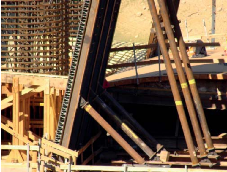
FIGURE 11.1 Custom pipe bracing.
