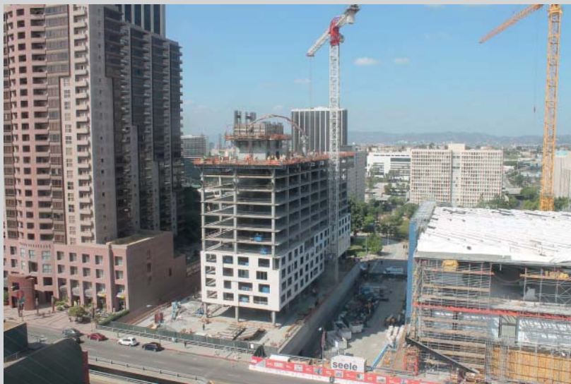
FIGURE 10.CS3 Twenty-story apartment building, Los Angeles, California (courtesy of Charles Pankow, Ltd and Doka Forms).
