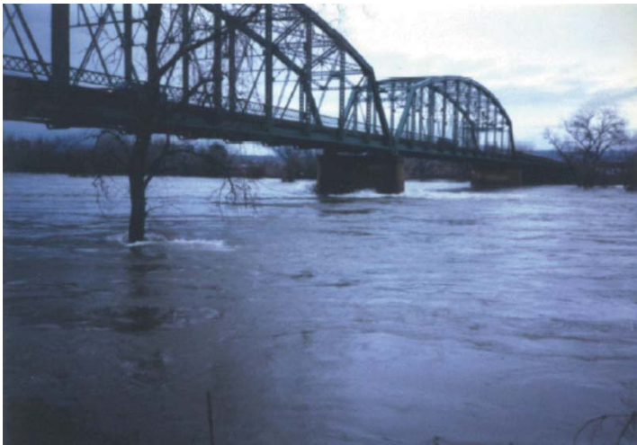
FIGURE 3.5 Flooding waters on a bridge pier.
