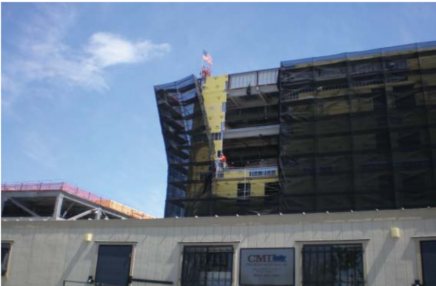
FIGURE 4.10 Scaffold connection to building failure.
