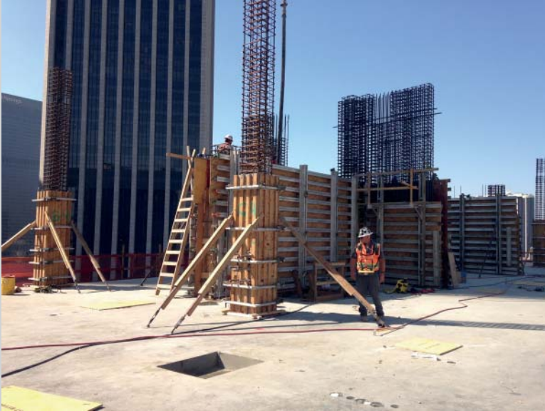
FIGURE 10.CS8 Concrete gravity columns and shear walls (courtesy of Charles Pankow, Ltd and Doka Forms).
