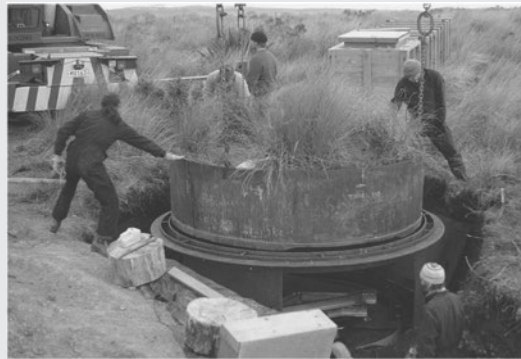
Figure 3.6 Large weighing lysimeter at Glendhu being installed. The weighing mechanism can be seen underneath.
